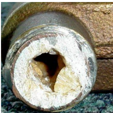
Hard Water Deposits in a Tap Water Pipe
